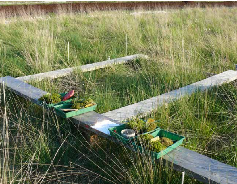
Sod transport and equipment for transplantation on an Eriophorum-Molinia site. The transfer of hummock moss sods requires thorough planning and preparation.
